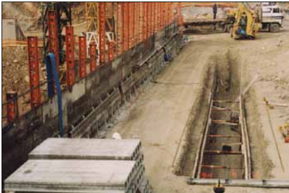
Figure 3 - Note pre-tensioned 150mm thick precast roof panels and 3m zone to upstream face
