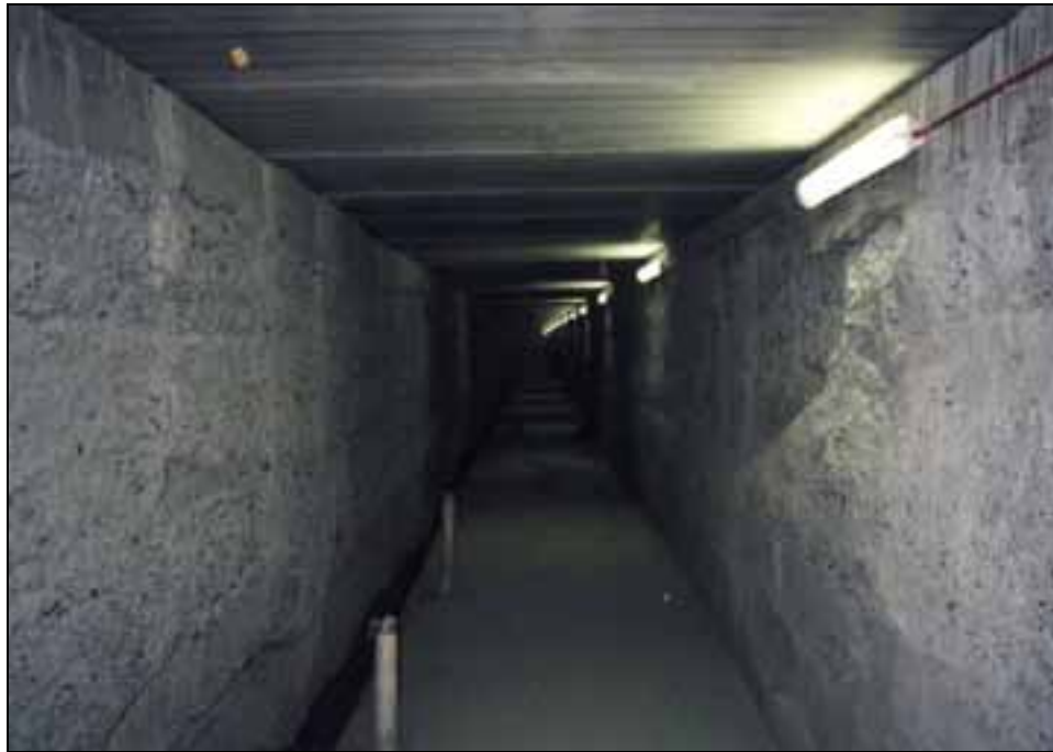
Figure 7 - Finished face of gallery with in-situ floor, drain holes and lighting fitted
