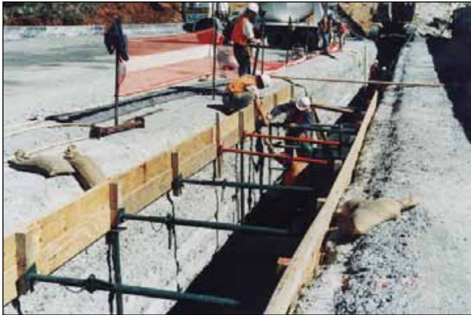
Figure 4 - Note truck delivering CVC to floor of gallery while excavation is proceeding at the top of the photo and forming of the sides continues at the base of the image
