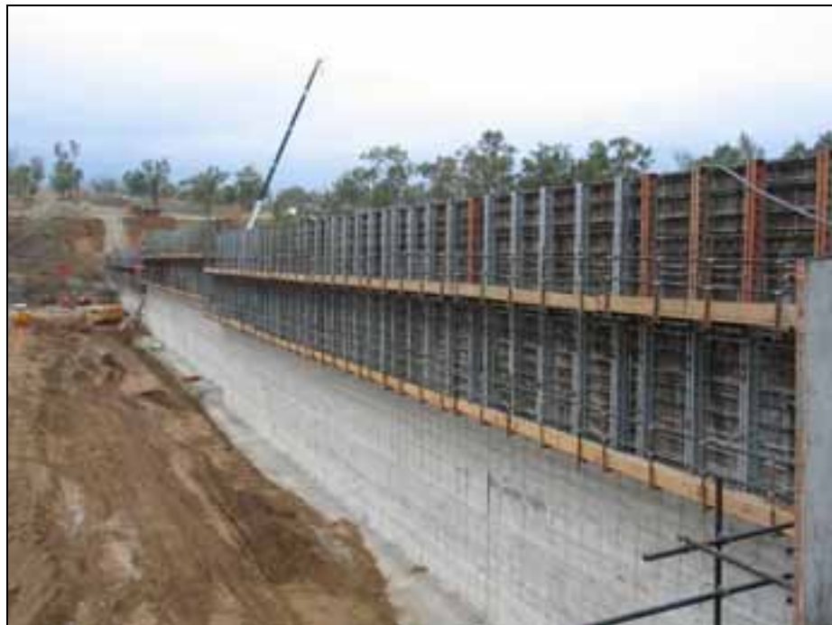
Upstream Forming of Eidsvold Weir using the Grout Enriched Vibratable RCC Process
